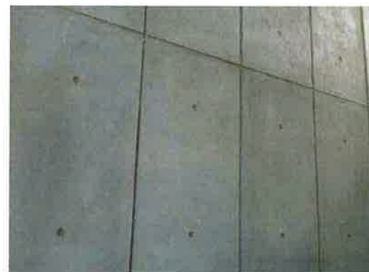
CONCRETE PANELS WITH FORMWORK HOLES
